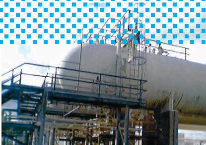
Horizontal cylinder tank
