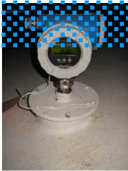
Levelflex M on top of the silo
