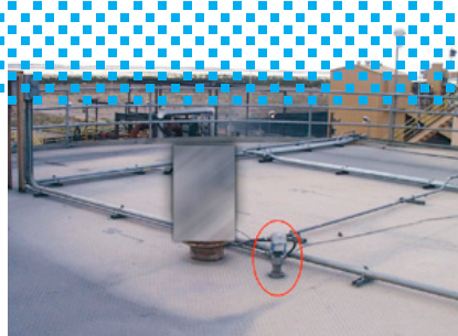
Levelflex installed beside abandoned mechanical device
