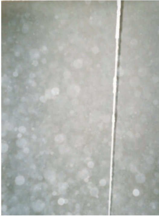
Fly ash build-up on the Levelflex cable inside the bin.
