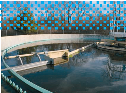
Aeration basin at wastewater treatment plant
