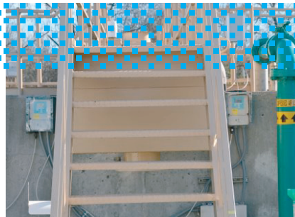
Two of the COM253 transmitters mounted on basin wall
