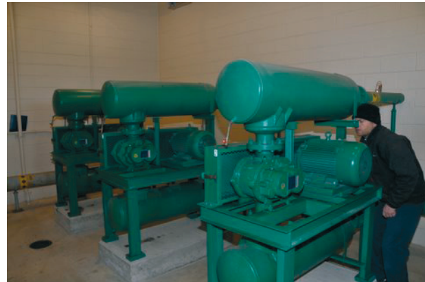
VFD controlled aeration pumps
